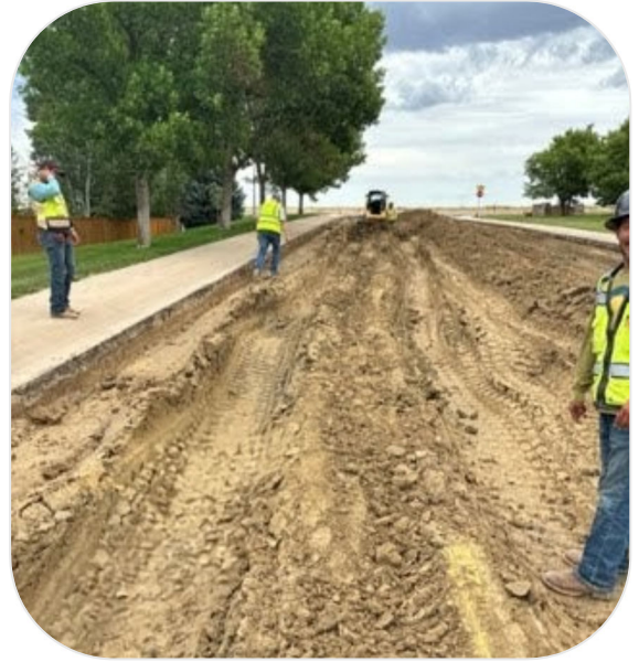
Before Mallard Drive Subgrade Repairs
