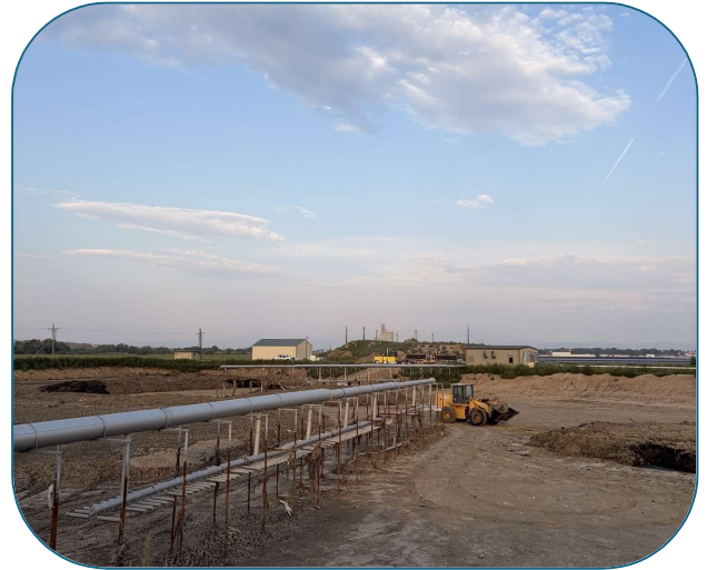
Lagoon Decommissioning Central Plant
