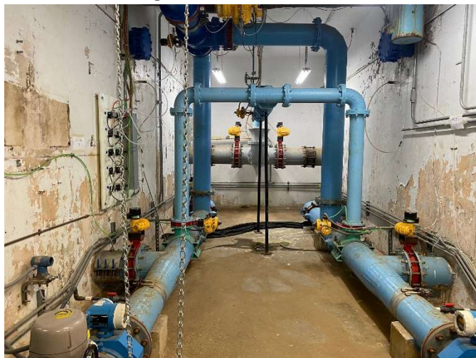
Photo: JWTP Existing Filter Pipe Gallery
