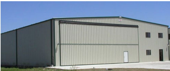
Figure 2-39 Unacceptable Metal Panel
