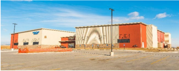
Figure 2-33 Unacceptable Metal Panel
