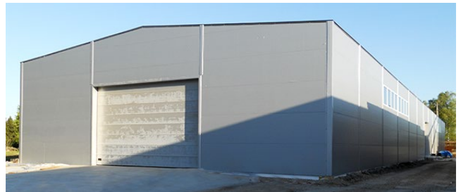
Figure 2-38 Unacceptable Metal Panel
