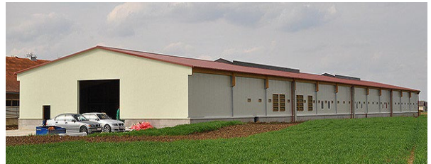
Figure 2-34 Unacceptable Metal Panel
