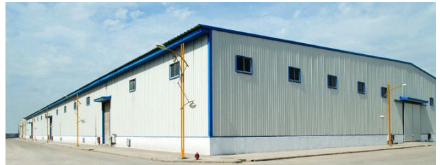
Figure 2-36 Unacceptable Metal Panel
