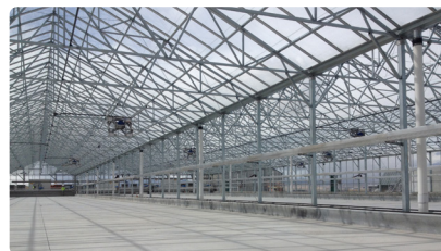
Tooele Solar Drying
