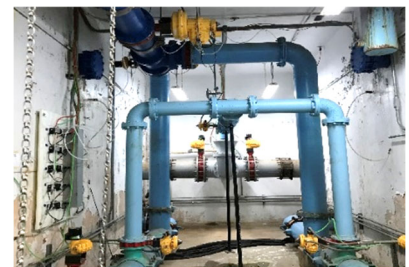
Figure 2-3. Existing Filter Gallery
