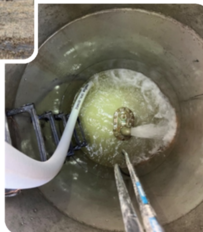
*Faulty Air Release-Vacuum Valve
