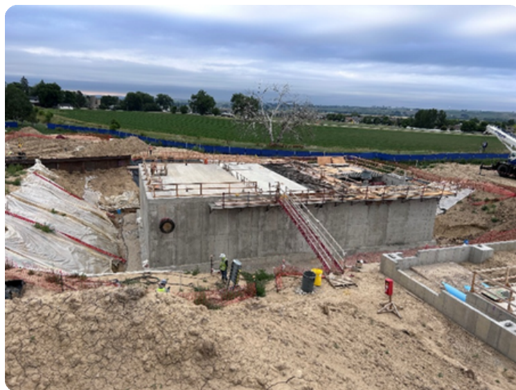
*Disinfection Contact Basin and Distribution Pump Station
