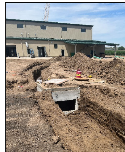
*Duct Banks Connecting New Buildings
