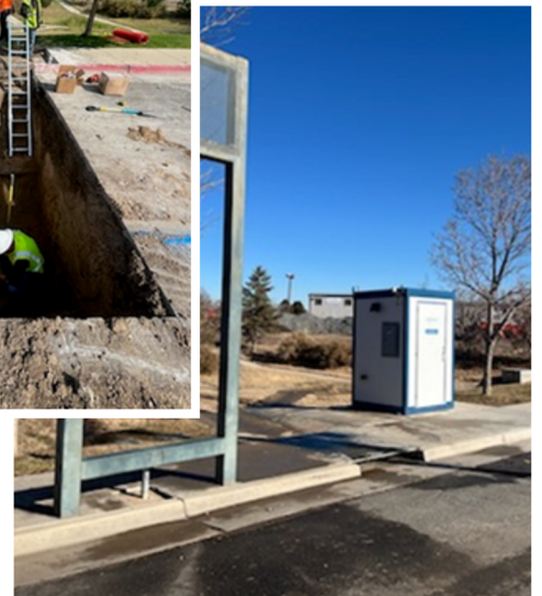
*New Bulk Water Station
