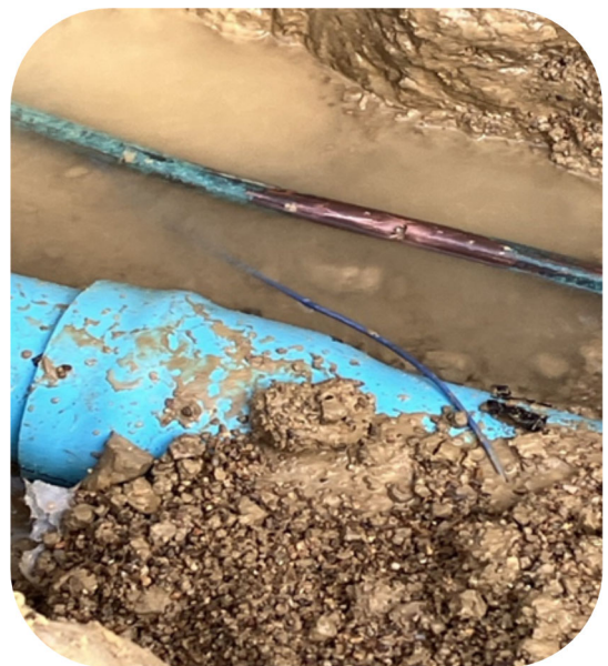
*Water Line Leak
