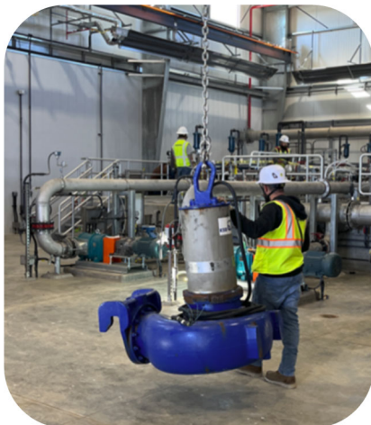
*New Return Pump at Central
