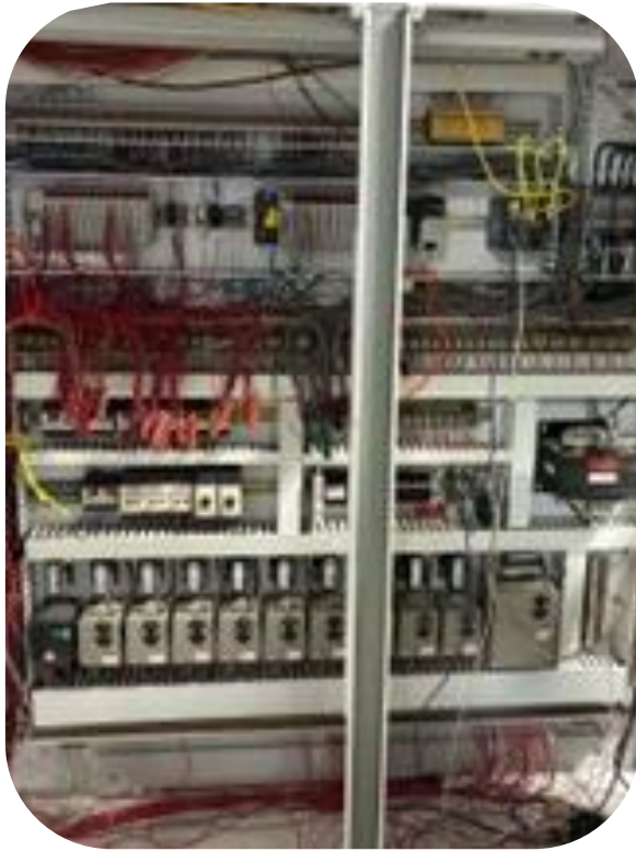
An Automation Cabinet Upgraded
