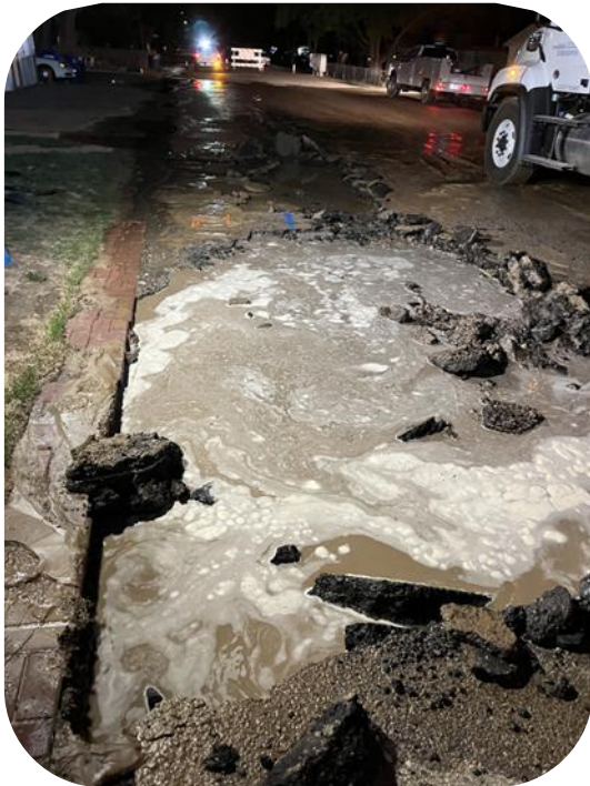
Water Main Break on S. 2 nd Street
